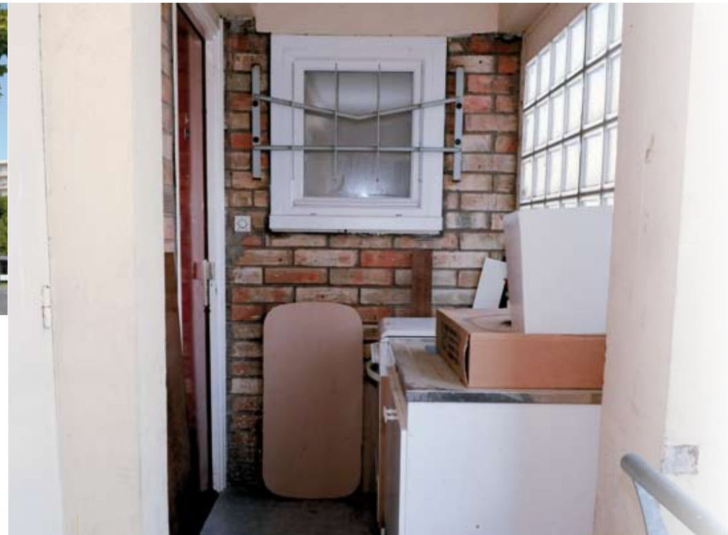
Palier encombré = danger !
